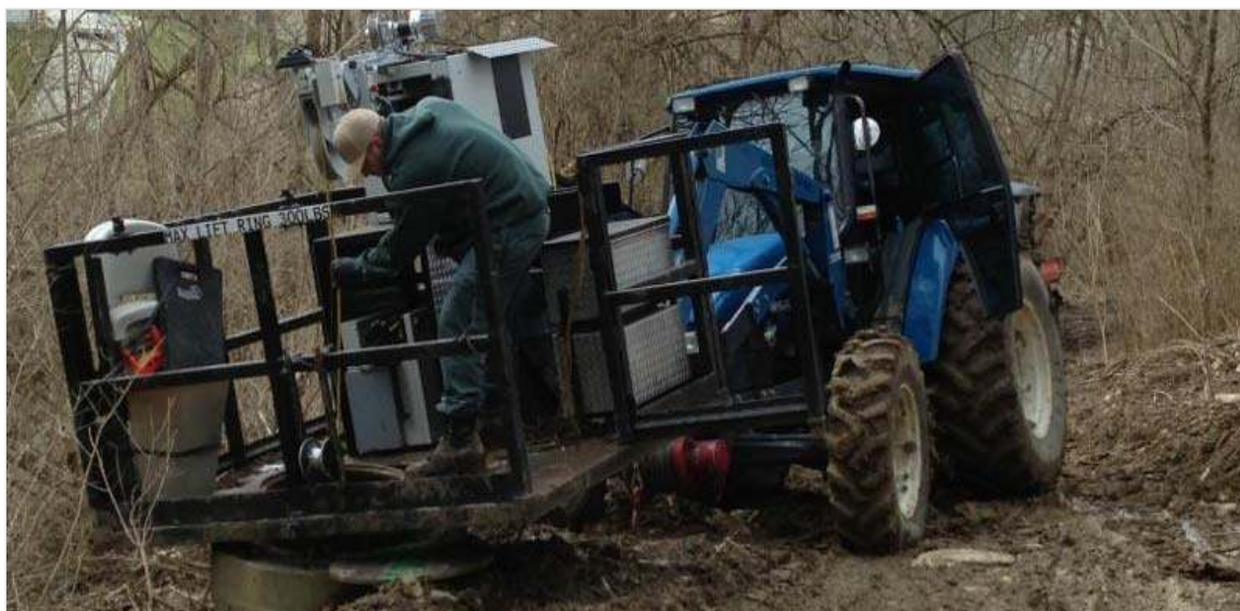
Figure 1-1. Custom Off-road CCTV Camera Tractor (Courtesy: MSDGC).
