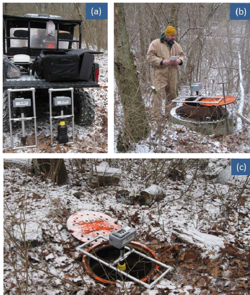
Figure 1-3. SL-RAT Deployment at EPA Project Site: (a) TX and RX Units in Transport Mode, (b) RX Unit Operational Mode Deployment, (c) TX Unit Operational Mode Deployment.
